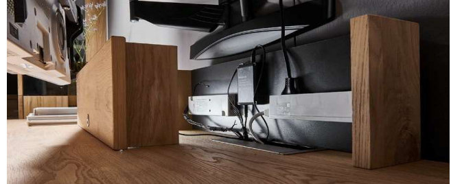
Fig. 2: Example of wiring
